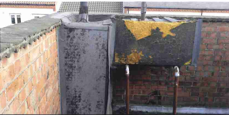
Before: Failed water tank housing. Leaking to upstands & pipework.
