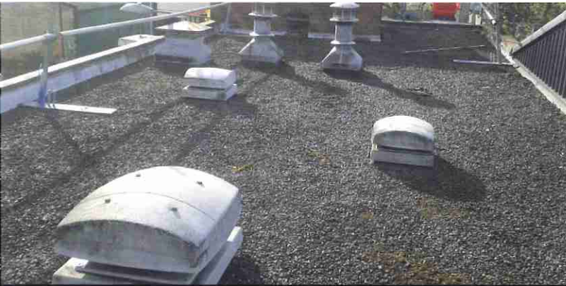
Before: Old felt roof with granite chippings. Leaking extensively.
